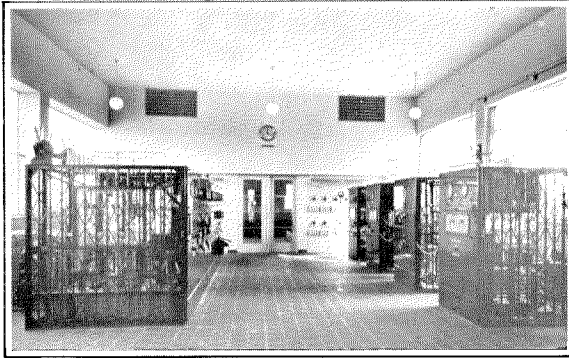
Figure 2—Transmitter Room Looking Towards the Machine Room at the Far End
